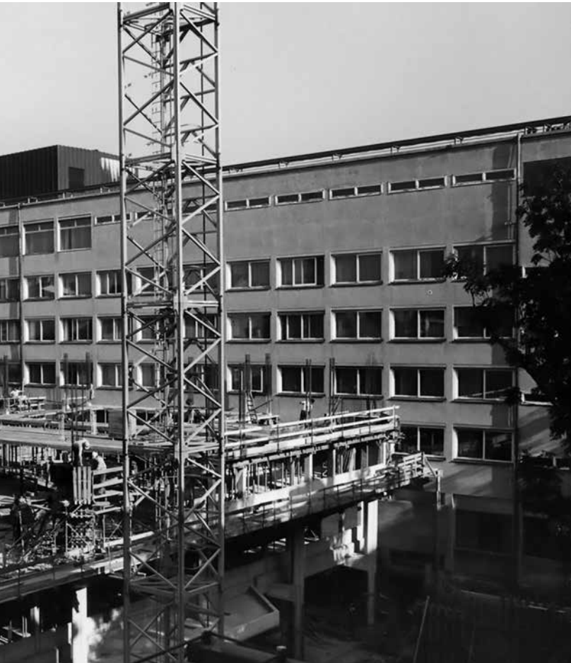
Construction of the Betriebs- und Sozialgebäude (BuS) in Munich-Schwabing, which housed the new Data Processing Center (DVZ) and the canteen of the head office.
